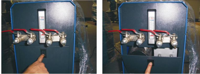
Picture 6-6: Pipe Heater 1
